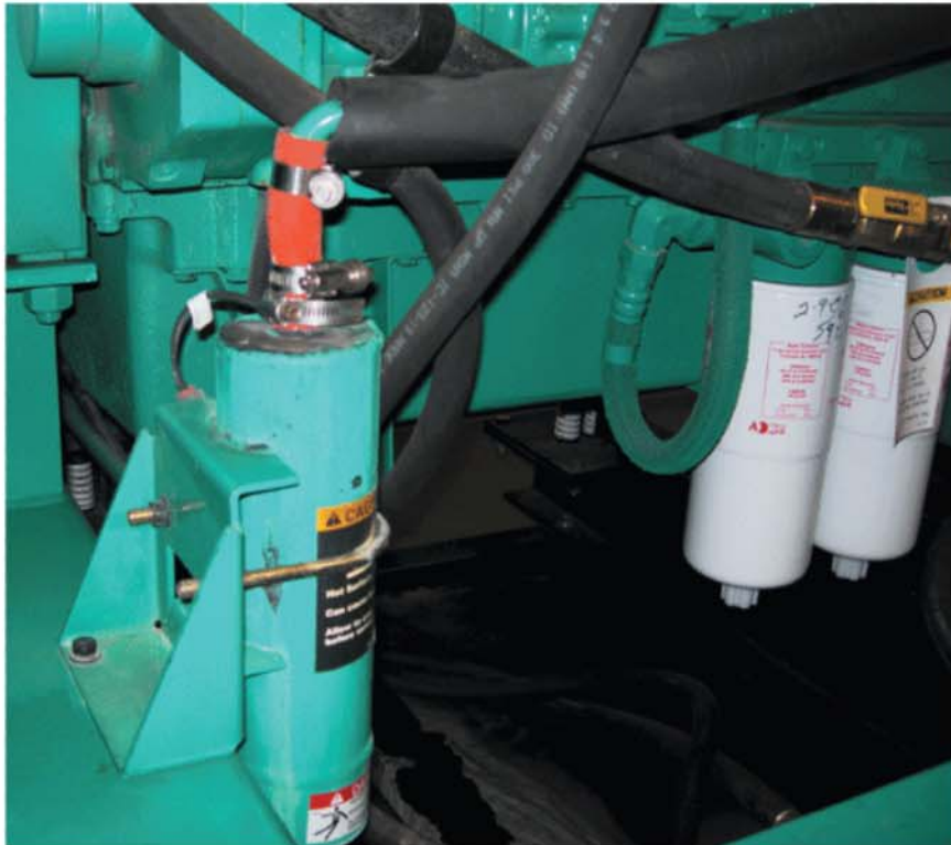
This shows one of two original equipment thermosiphon preheaters on a 1,500 kW genset. Photo: Kim Hotstart
