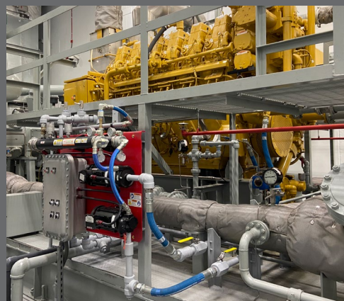
Photograph of the experimental setup at the Miami Lakes Learning Center (MLLC). This setup is intended for experimental purposes and is not to be used as a recommended design practice.
